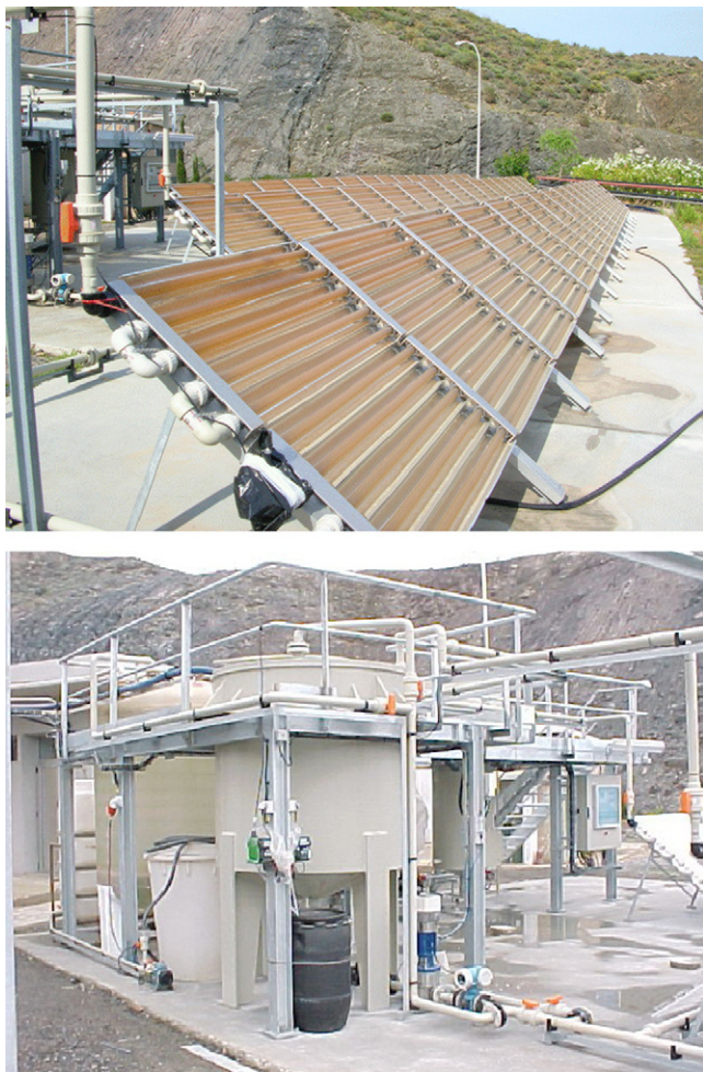
Fig. 5. Views of the industrial plant: CPC field (up), tanks and P&I (down).
